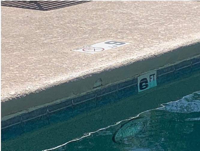
Pool decking delamination
