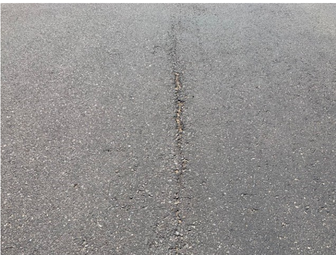
Isolated asphalt cracks
