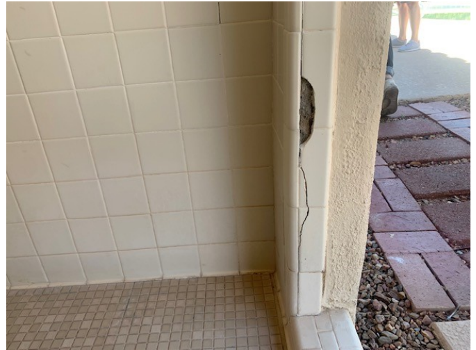
Cracked tile (A)
