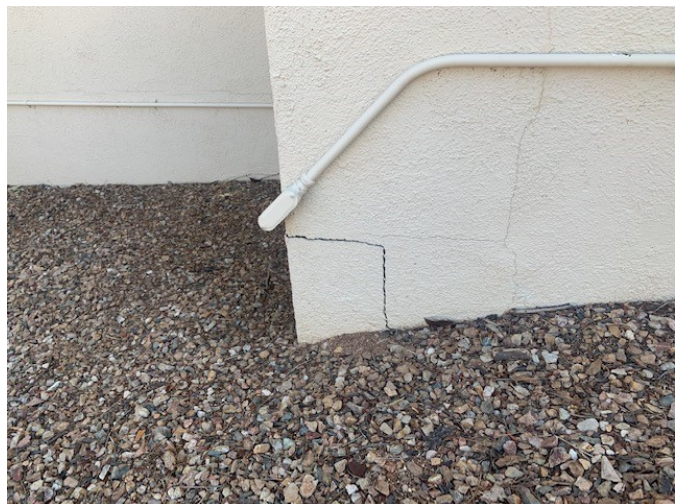
Crack in wall
